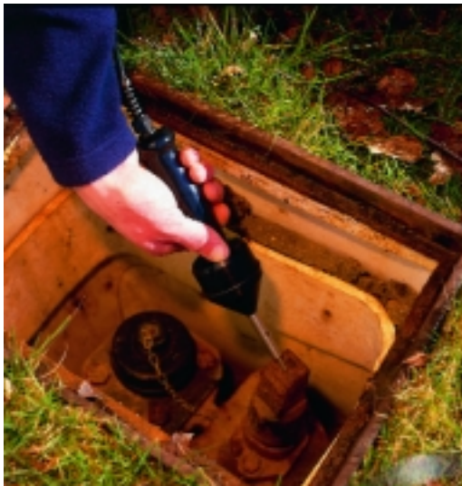
Listening at hydrant using the hand probe
